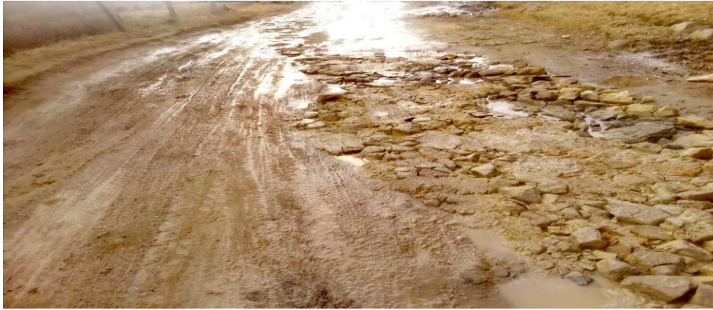
Image 4.8.2(b) A dirt road in MASOWE
