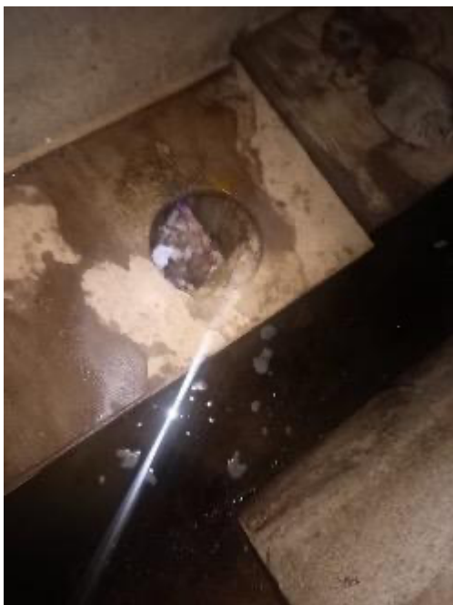
Figure 3: Visual depiction of the condition of toilet facility
