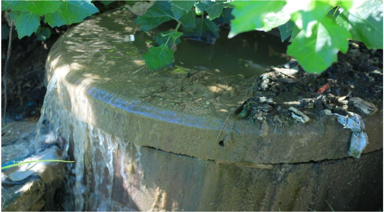
Figure 1.1: Location of Leaking Sewer Line at 29.8 0 S, 27.4 0 E (source: Motaung and Mahao, 2025)
