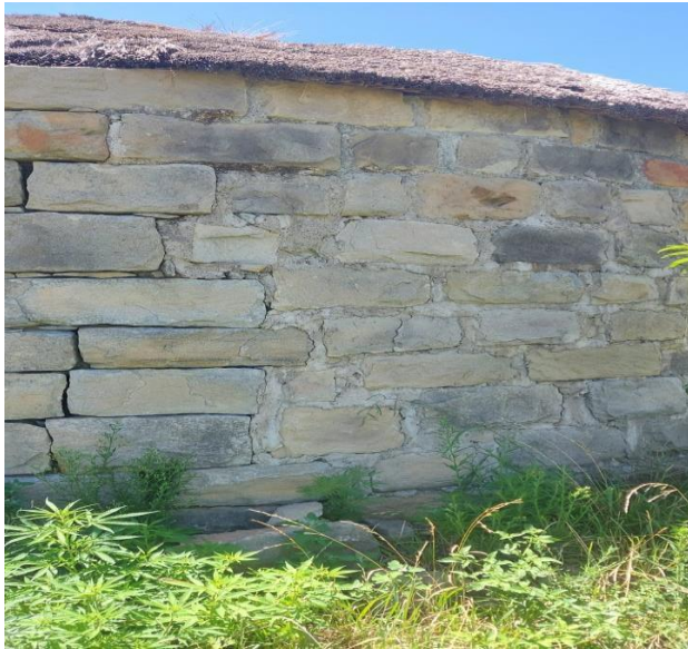
Picture: Structure affected by aggregate mining at Ha Tikoe
