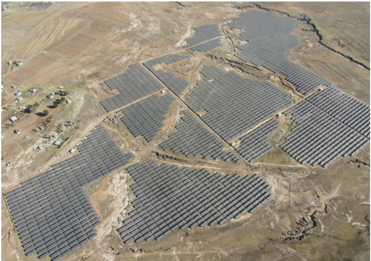
Figure 7: Ramarothole ground mounted solar panels.
