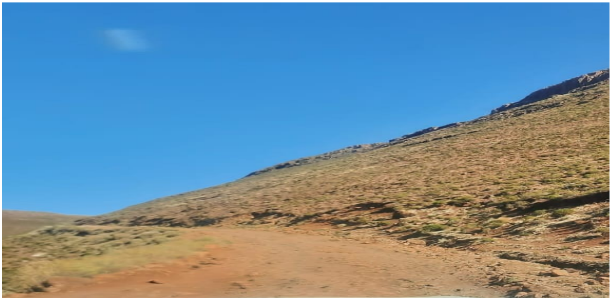
Figure 4.3: The local road’s vulnerability to erosions
