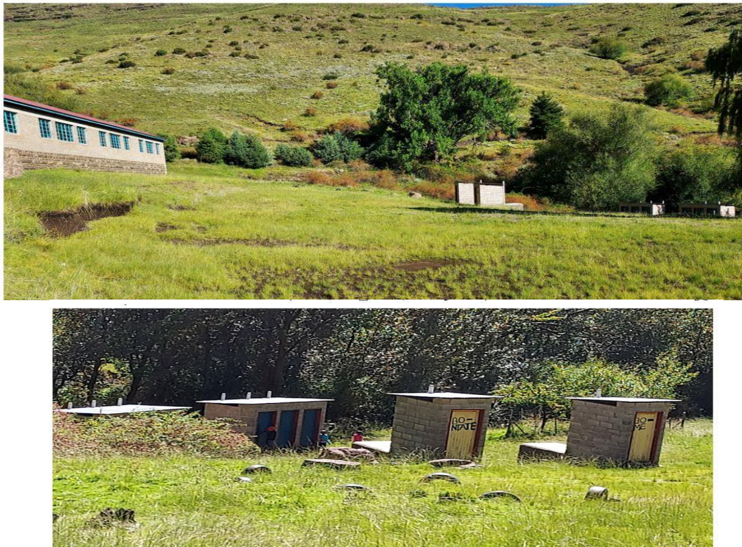
Figure 5: VIP Toilets at St. John the Baptist Primary School
